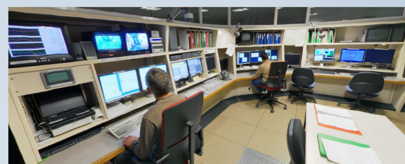
WHT control room
