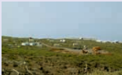
MAGIC foundations close to the former HEGRA site with the Residencia in the background.
