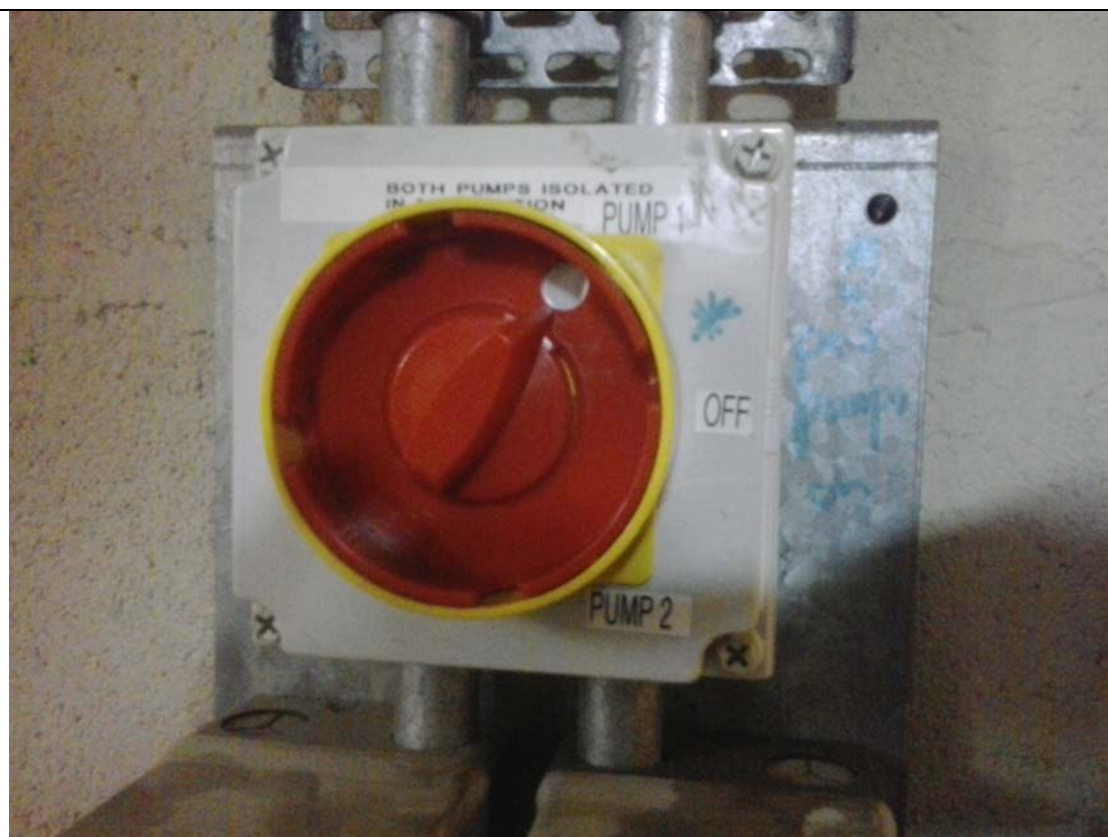
Figure 3 Oil pump power switch
