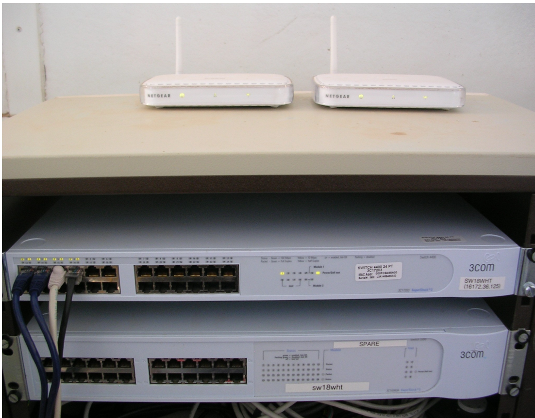
Picture 6 wireless access point + hubs mounted in dome wall box 1
