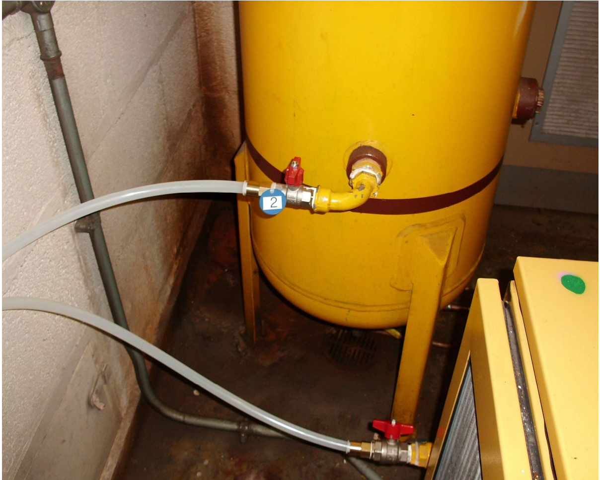
Valve 2 1/2" inlet to the storage tank.
