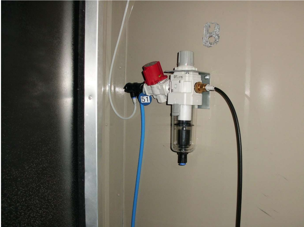
Valve 51 of air supply to the Ghril door
