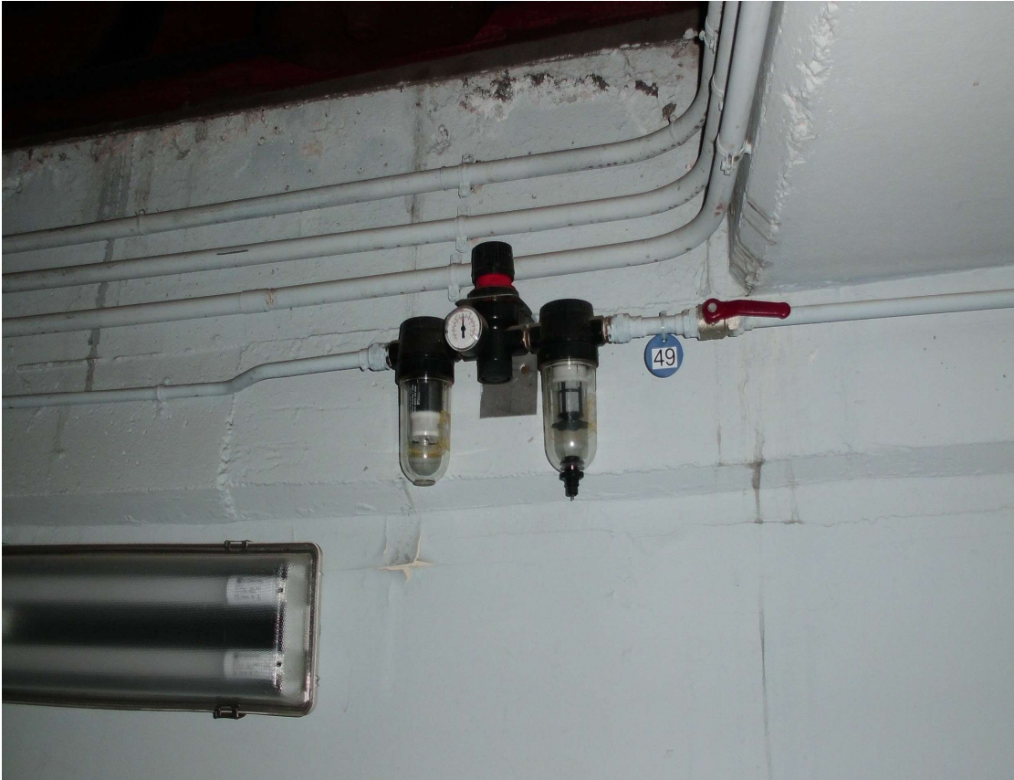
Valve 49 of air supply to the observation floor area of Cassegrain and rolling hose.
