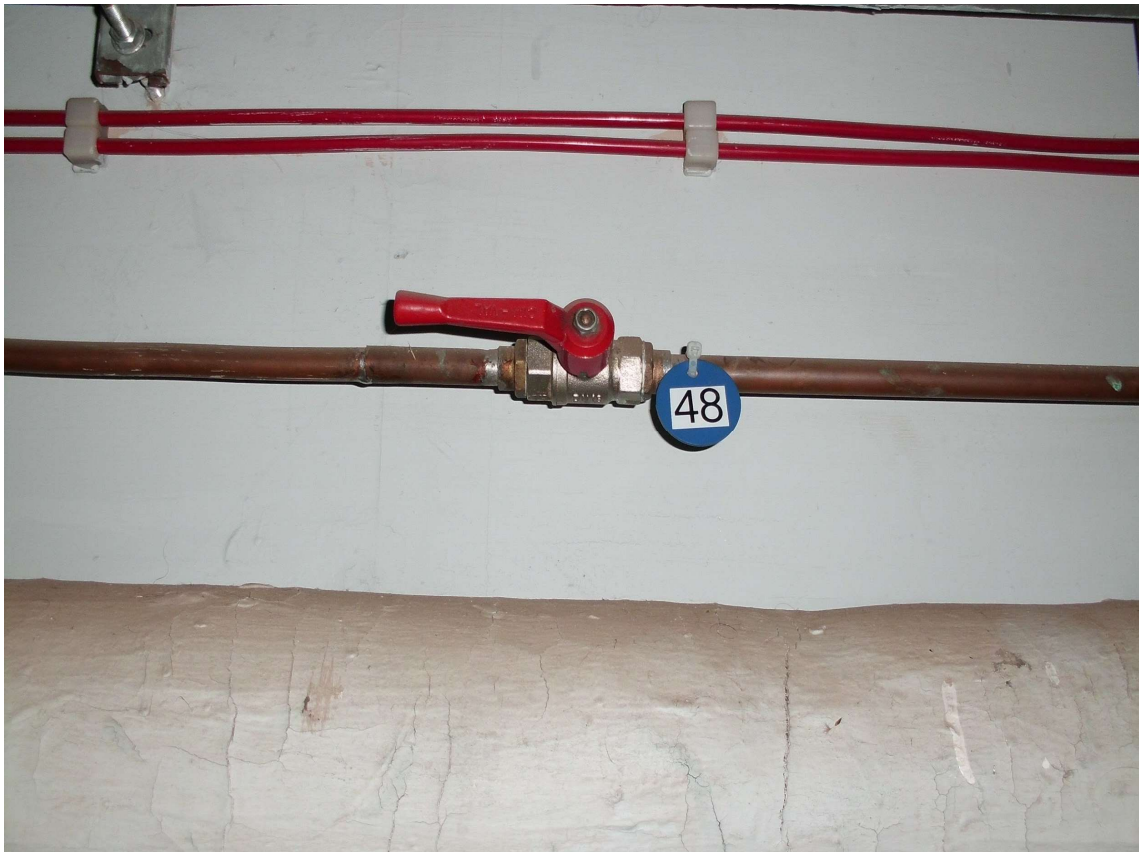
Valve 48 for air supply to the dome corridor from the base corridor of the WHT.
