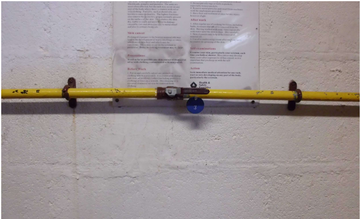
Valve 3 of 1/2" from the accumulator tank.
