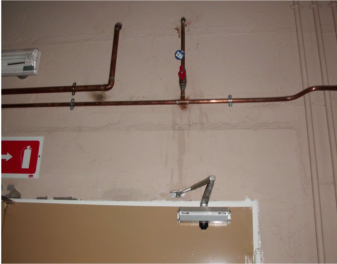
Valve 47 for air supply to the Detector Laboratory on the 2nd floor.
