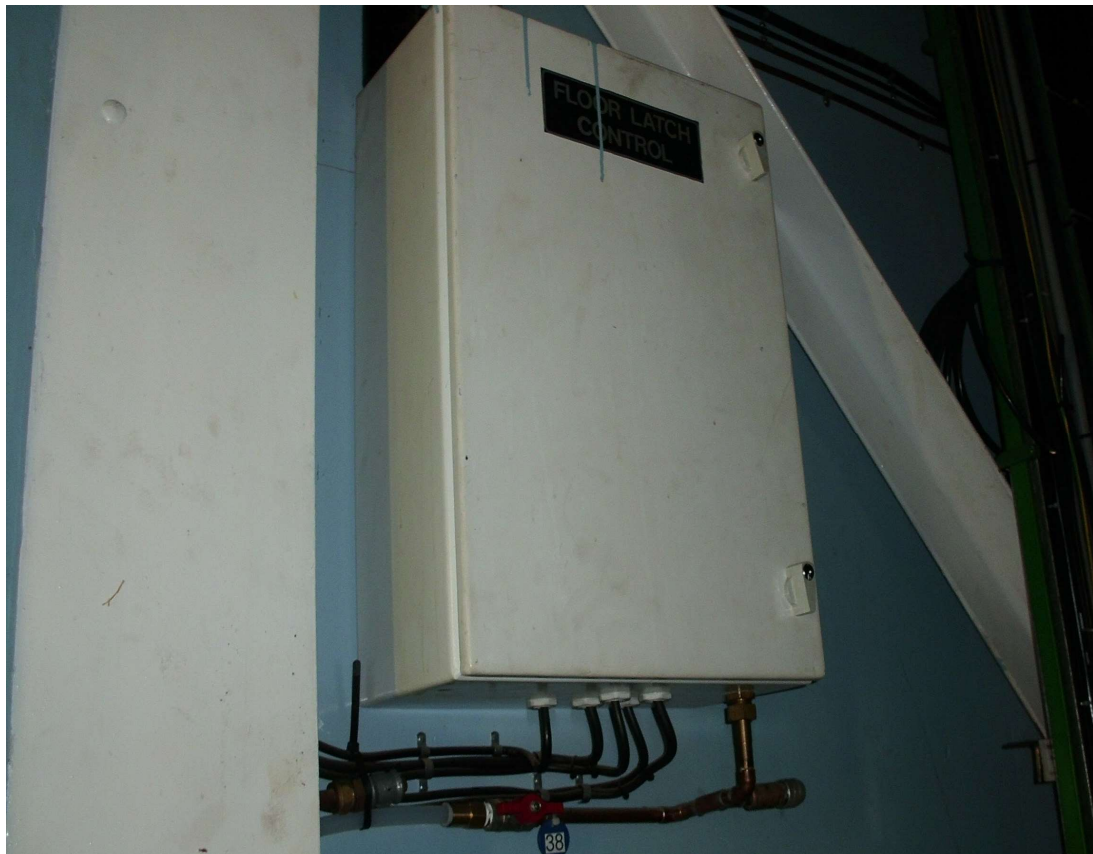
Valve 38 for supply to the Floor Latch Control System in the entrance area to the Azimut movement.
